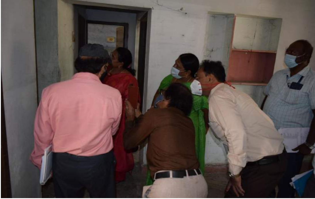
Structural Damage Assessment of Dilapidated 54 Nos. of TNGRHS Flats at Moolapalayam, Erode
